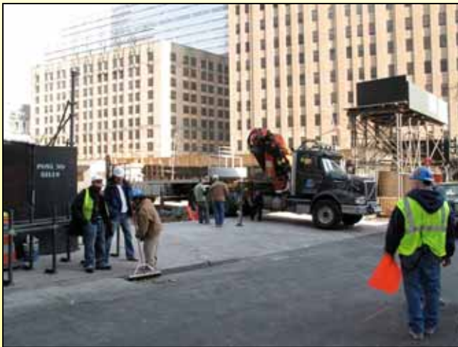
Example of Engineering Control: Workers sweeping track-out for dust control at Goldman Sachs construction gate
