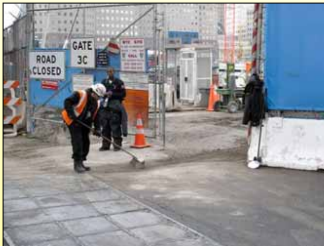
Example of Engineering Control: Workers sweeping track-out for dust control at World Trade Center construction gate
