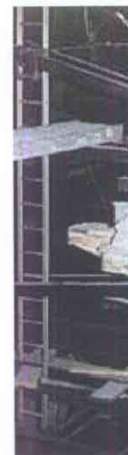
New steel to vertical colu supporting c slabs by the BY BRYAN
